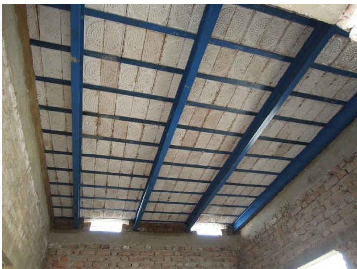
Completed ceiling with T-bars, iron T-profiles and roof tiles including ventilation openings.
