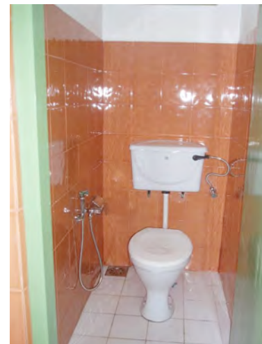
Building D: Teacher toilet
