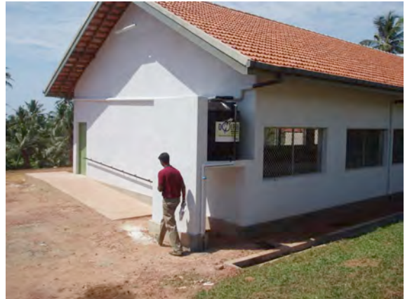
Rain water harvesting system for building A, B, C & D 5 tanks with 1000lt
