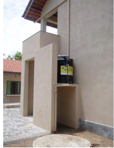
Rain water harvesting system 8 tanks with 1000lt
