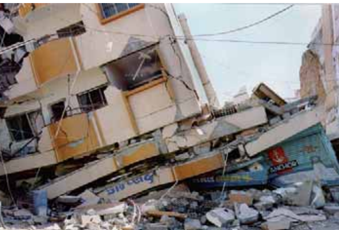
Earthquake damage in Bhuj, India (2001)
