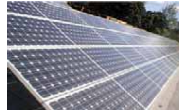
Photovoltaic panels, used to produce electricity
