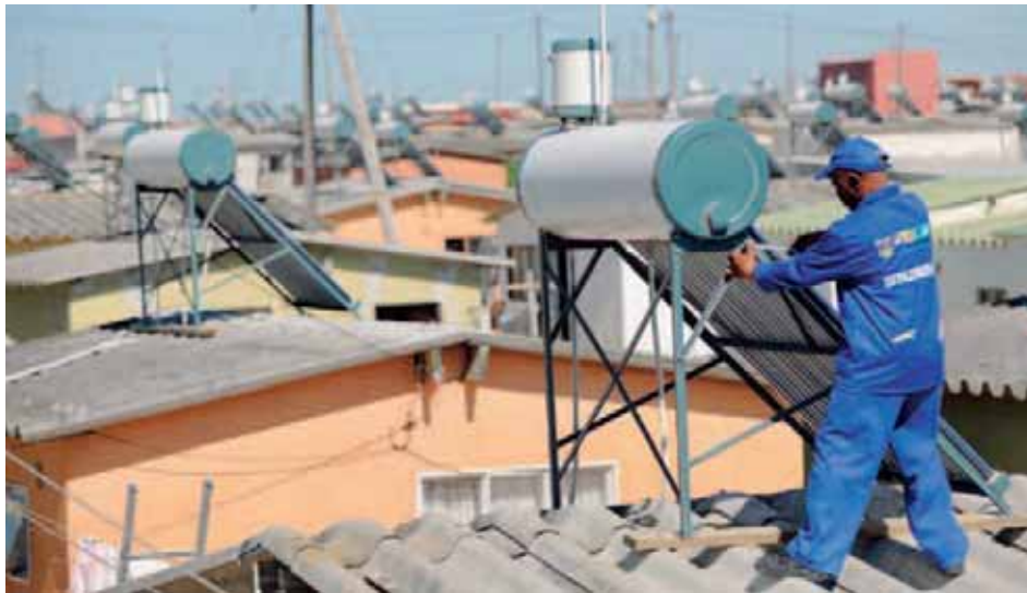
Solar panels for hot-water production in Bruce Sutherland, City of Cape Town 61
