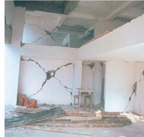
Image 17 : X (cross) Shaped Cracks
