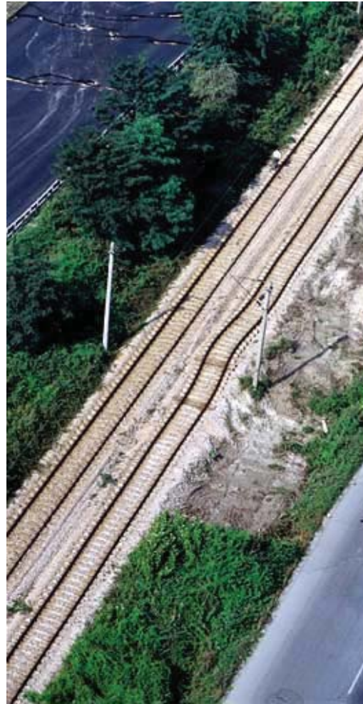
Image 10 : Damages to Man-made Structures, Izmit
