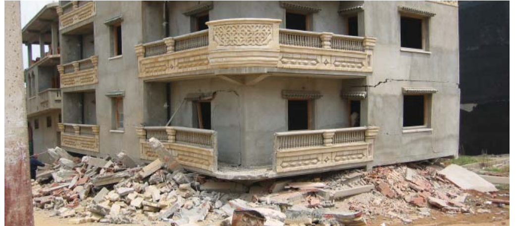
Image 13 : Soft Story, 2003 Boumerdes Earthquake
