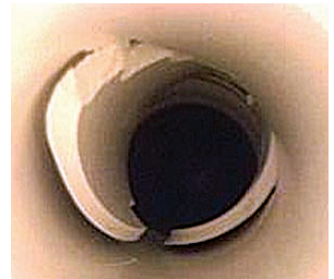
Figure 18: Casing damage as seen through a borehole CCTV camera
