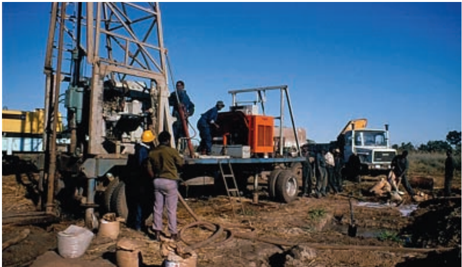
Figure 2: A mud rotary machine working in eastern Zimbabwe, 1996. Note the mud pits dug nearby
